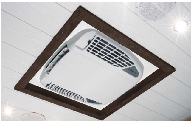
Klimaanlage, Decke Air conditioning, ceiling
